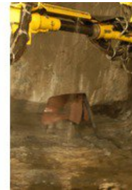
KRS-Pump in a cage, protected against rockslide
