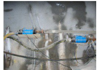
Horizontal Pumps: "Horizontal booster pumps in the Bleßberg Tunnel"
