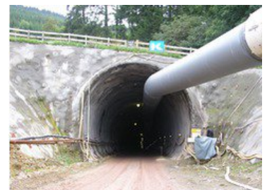
900 metre stretch of pumping in "The Bleßberg Tunnel: chains of pumps reaching 900 metres and more are possible when connecting pumps in series"
