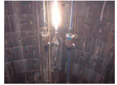
Vertical Pumps: "Riser pipes in the supply shaft: Four small Tsurumi pumps installed in series are all that's needed to ensure drainage vertically upwards through the tunnel"
