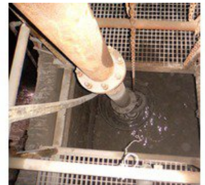
Pump sump with a riser: more than 100 pumps from Tsurumi are used to pump water in the mine (Photo: Tsurumi) Download photo
