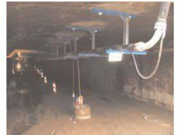
Support of the drain line by a pipe bridge, 2nd section of excavation.
