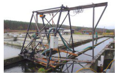
Pump instead of excavator: The channel with pump at the front and the tank where the sludgy problem comes from behind. The channel had to be dredged once a year up until now (photo: Tsurumi) Download photo
