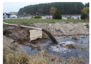
The sludgy mixture is channelled through a hose to the sedimentation tank (photo: Tsurumi) Download photo
