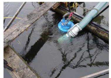
The submersible pump hangs on a chain, meaning it can be freely positioned (photo: Tsurumi) Download photo
