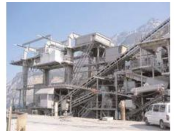
View of the grab dredge plant with parts of the transport system
