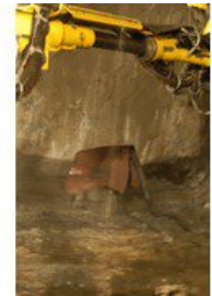
KRS-Pump in a cage, protected against rockslide
